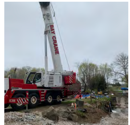
Site activity during April 2022, the first month of Phase 1 repairs on the north side of the dam. Photo credit Craig Wood.
