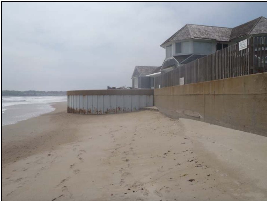
Figure 9. Seawall and sheet pile bump out protecting private properties near the center of Narragansett barrier spit.
