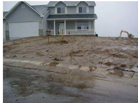
Example of erosion from a construction site.
